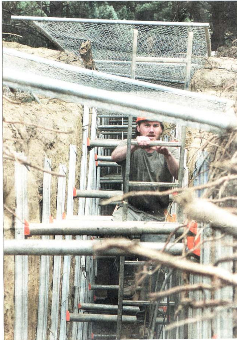
Geologist Todd Becker ascends from a trench on the College of the Redwoods campus. Laco Associates is digging and checking several trenches to search for active faults that may determine where new structures are located. See additional photo on Page A8.
